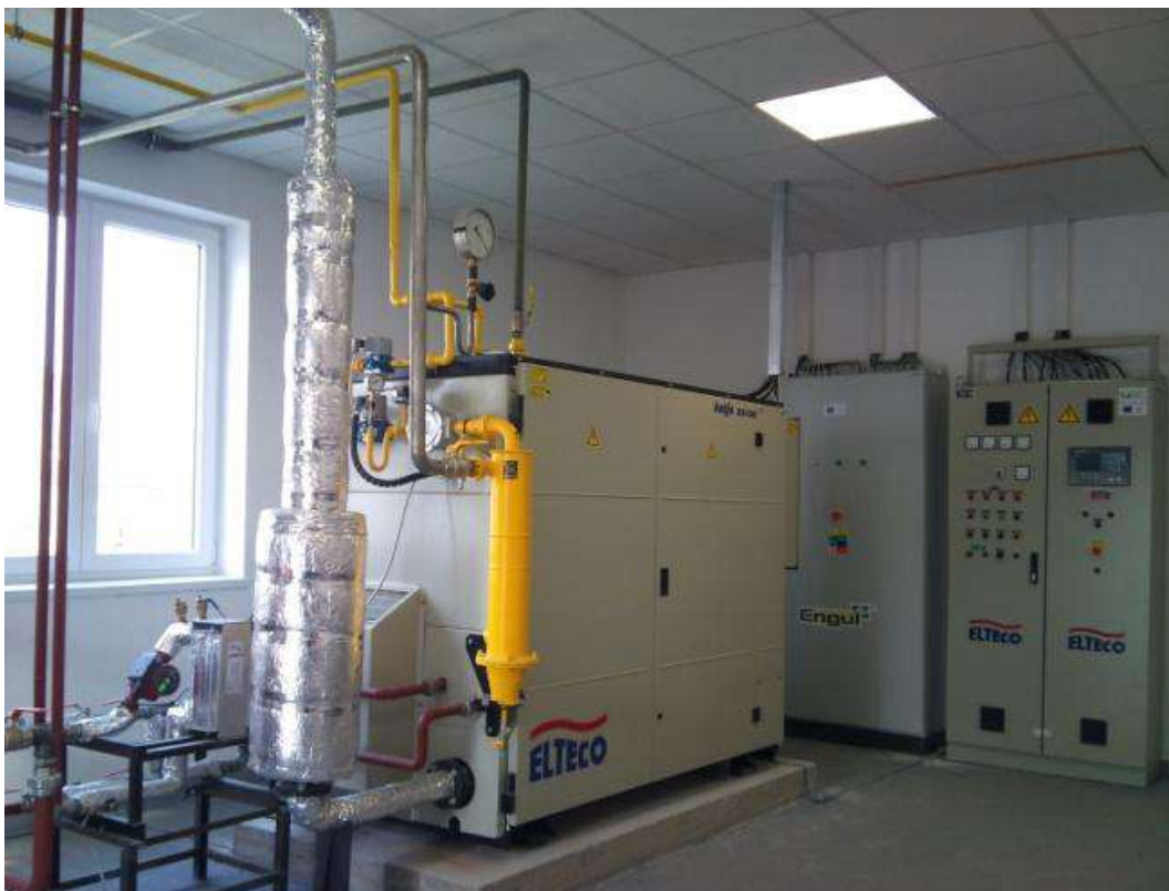
Fig. 3 Existing cogeneration unit – source of technological heat and biogas burner
