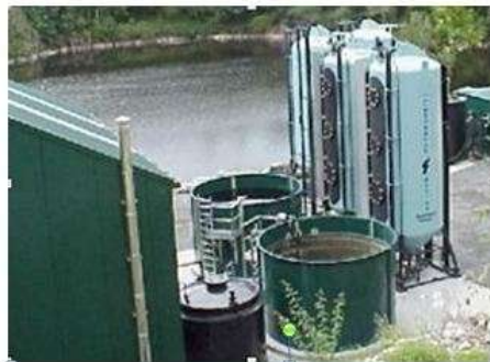
Figure 4: Activated Carbon Filter for As- Removal
