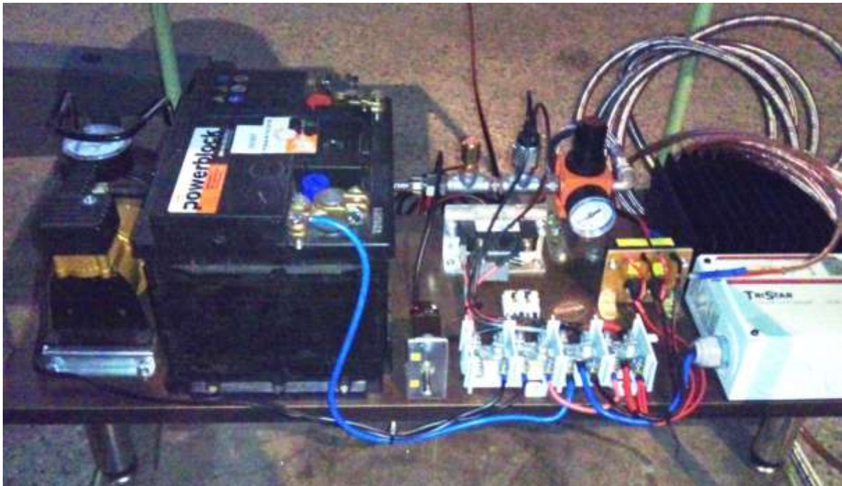
Fig.3 Module of source of compressed air, battery and charging controller
